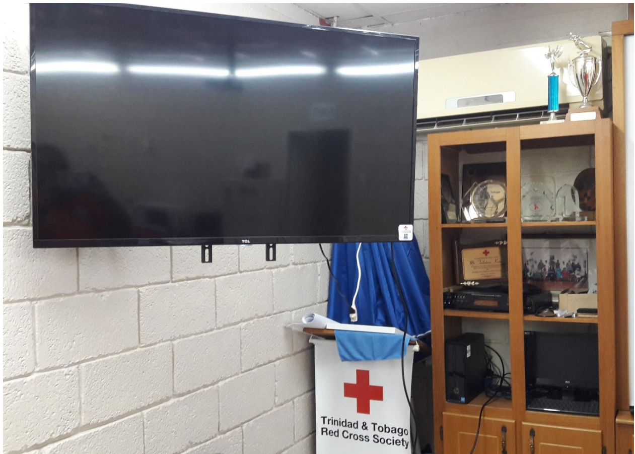
Figure 4: 50" Monitor and Computer installed at TTRCS Conference Room which is used during emergencies as the EOC, this computer system lets us monitor the FEWS software in real time.
