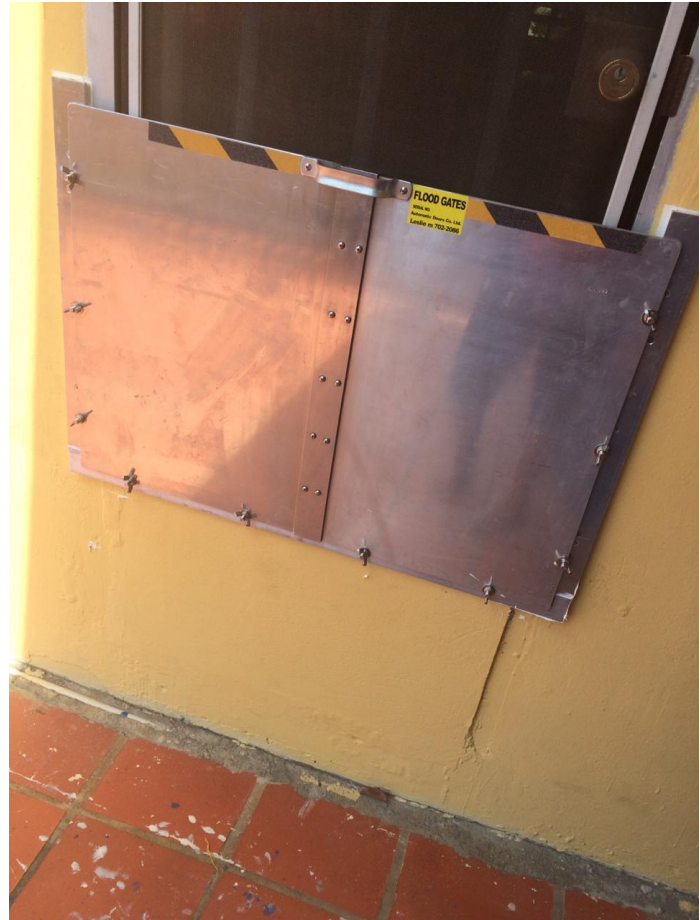
Figure 5: One of the Flood gates installed at the old-age home, St. Helena.
